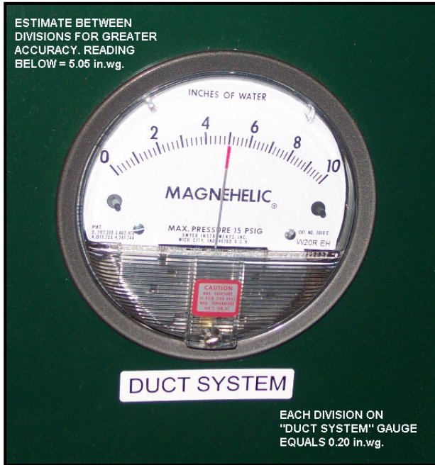
Figure 14 – Duct System Gauge Pressure Reading
